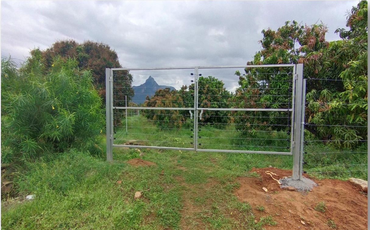
Fig. Fixed Type Solar Fencing system installed in the farmer's field at Vallakundapuram in Tiruppur District of Tamil Nadu
